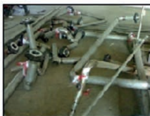
JANA-SS Piping Spools
