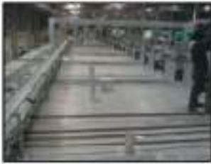
Gulf Packjaging-Thermovel Oil Piping
