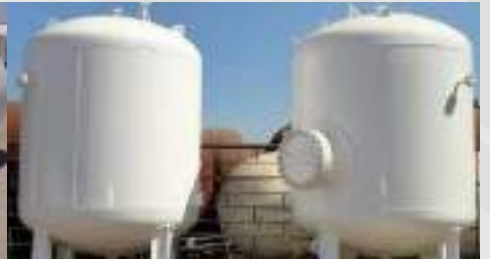
3) VERTICAL LPG TANK
