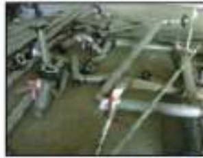
JANA-SS Piping Spools
