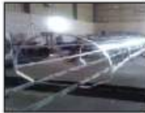
Dehran Tower-Aluminum Cat Ladders 700 LM
